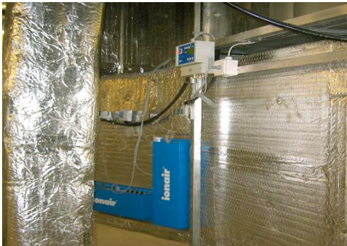
Installed Ionair® system with ICE/A Controller
